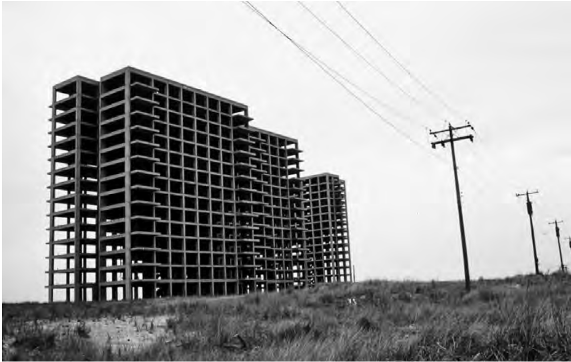
Abandoned apartment building skeleton on the Breezy Point peninsula, NYC. Photo by Arthur Tress/NARA.
